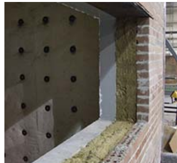
Thermafiber ® Safing Insulation in jamb and sill with continuous steel lintel at head
