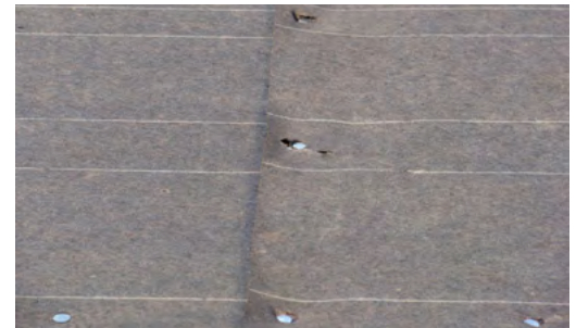
Standard felt tears and curls away from fasteners after exposed to moisture.
