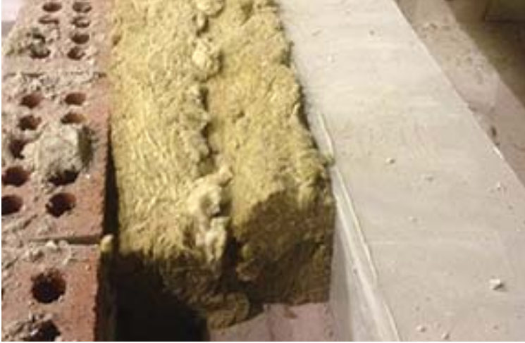
Figure 2: Correct compression installation around an opening in a wall with masonry veneer over CMU structural backup
