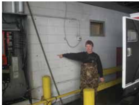
➤ During the damage assessment phase, Bill Dowd points to the water level reached inside the plant.
