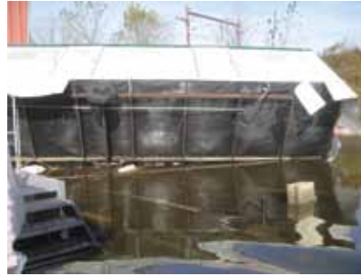
➤ The shipping trailer on the asphalt side of the plant was overturned.
