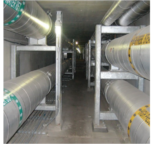
Insulation systems in vaulted or tunneled applications must be able to withstand potential flooding, limit risk to other assets and protect pipes from maintenance traffic or burrowing vermin that could cause damage.
