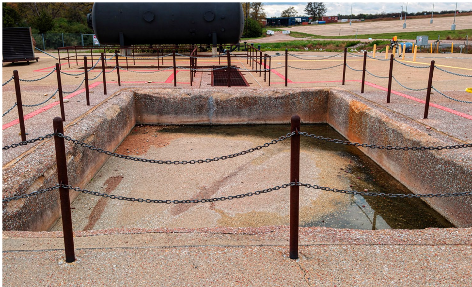
Figure 3. The LNG impoundment.
