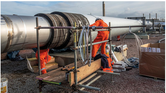
Grain LNG, UK, a two-layer, no-contraction joint, all-FOAMGLAS® insulation LNG piping insulation system.
